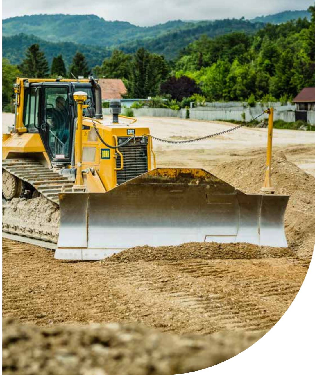
Flood retention basin Fahrafeld/Lower Austria – Austria Earthworks at the largest retention basin in Lower Austria
