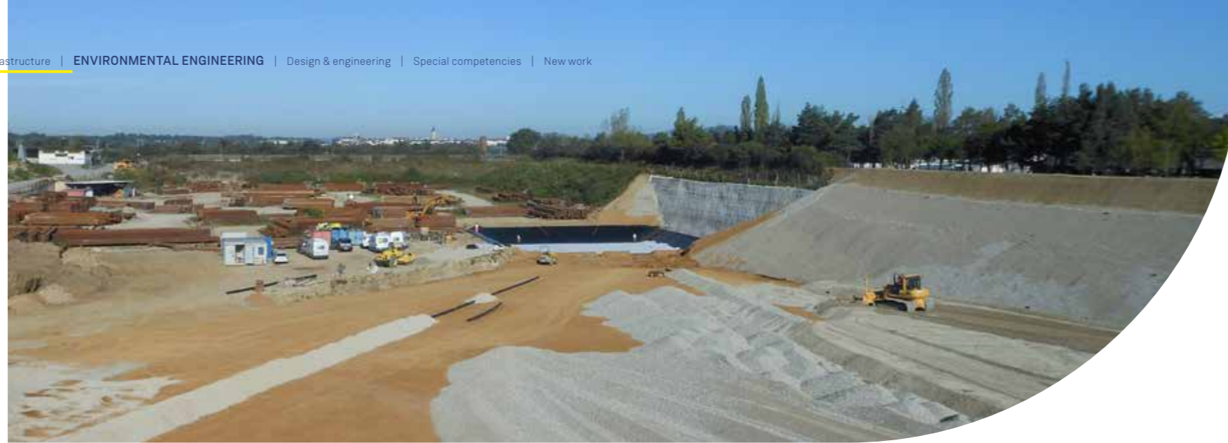
Rems construction waste landfill and recycling plant – Austria State-of-the-art storage for numerous types of waste
